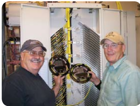
Splicing contractors inspect the ADC OMX600 splice cabinet after installation. ADC's patented splice wheel design maintains bend radius and ensures limited congestion
