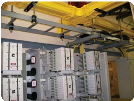
ADC FiberGuide provides the overhead cable management for the NGF fiber termination frames in a KPU Central Office
